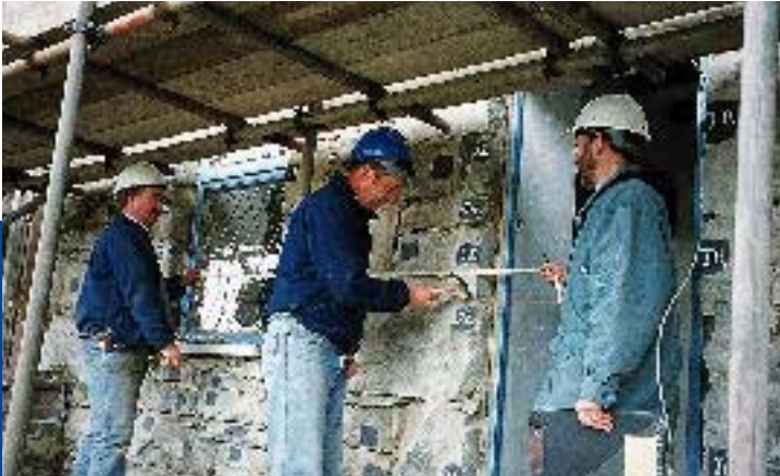
Staff from the Museum of Welsh Life dismantling the Fron Haul row of quarrymen's houses, ready for re-erection at WSM.
