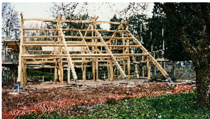
The Welsh oak framework of the house shows how this building looks forward to the future on the basis of traditional building techniques.
