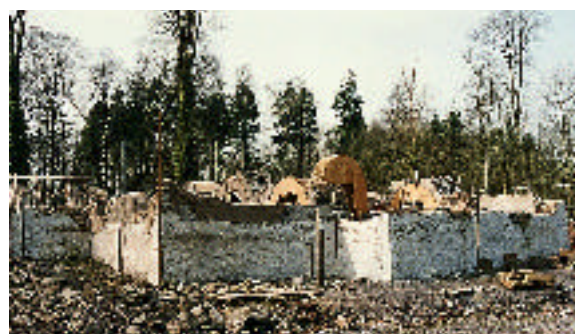
St Teilo's Church, from Llandeilo Tal-y-bont, being re-erected at the Museum of Welsh Life.
