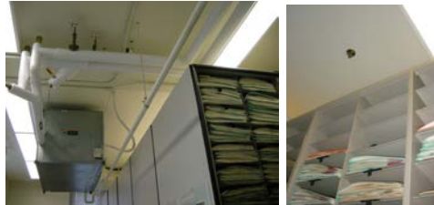
Photographed by Nicholas Wojtas Open concept compactor system showing potential sources of overhead water damage.
